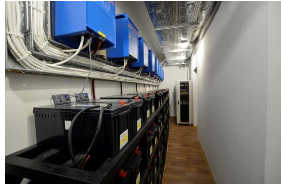
4 Nine Victron Energy power units
