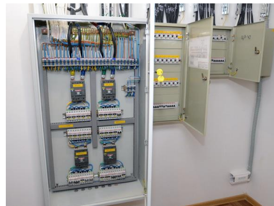
3Parallel isolation system for individual units allows any unit to be isolated for maintenance without shutting down the system
